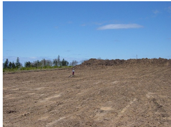
Judith Peach standing in cleared turbine site #13, Digby Neck Wind Farm - See story next page
